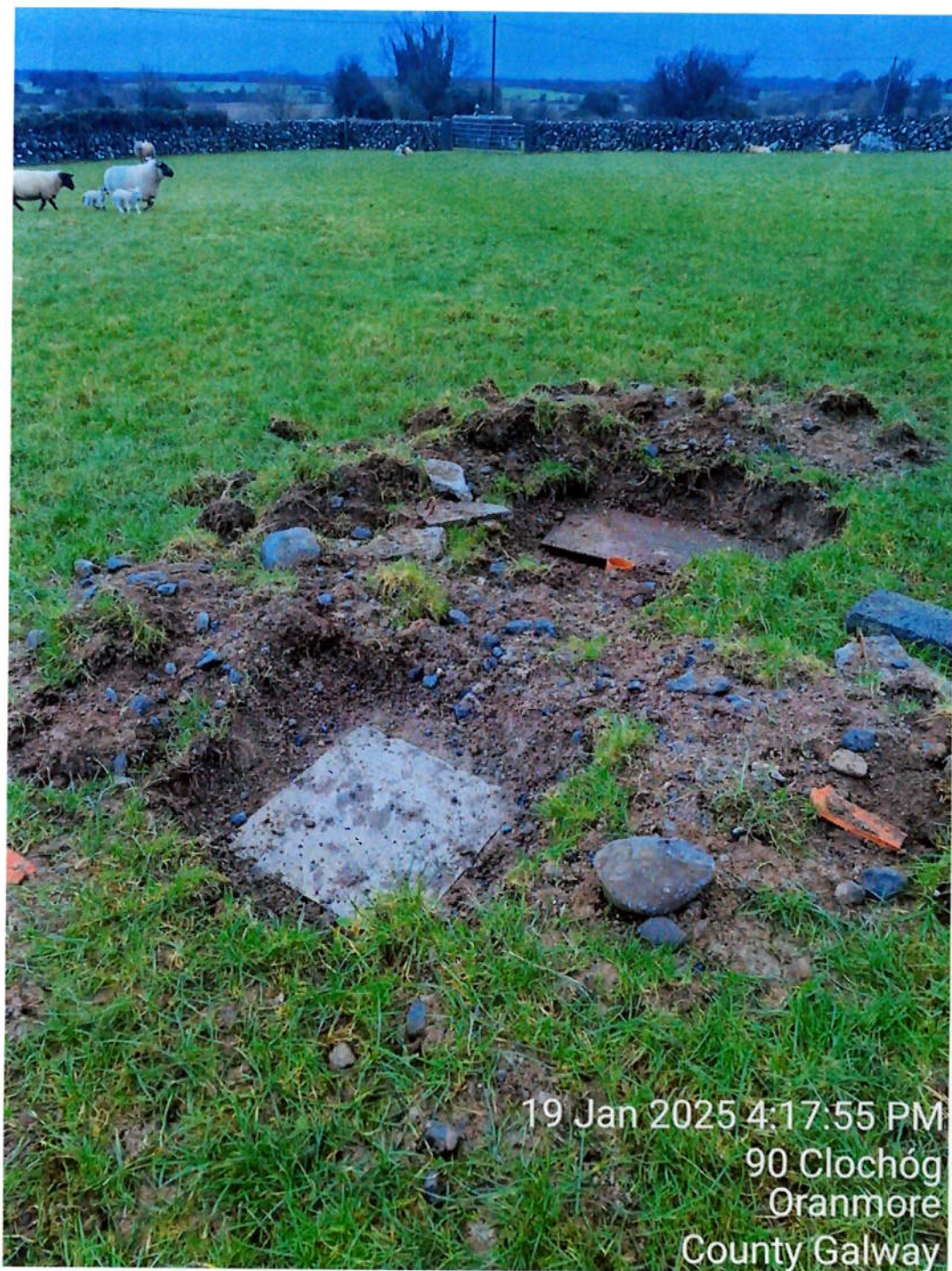
Fig 02. Photograph of exposed septic tank – location as per drawings
