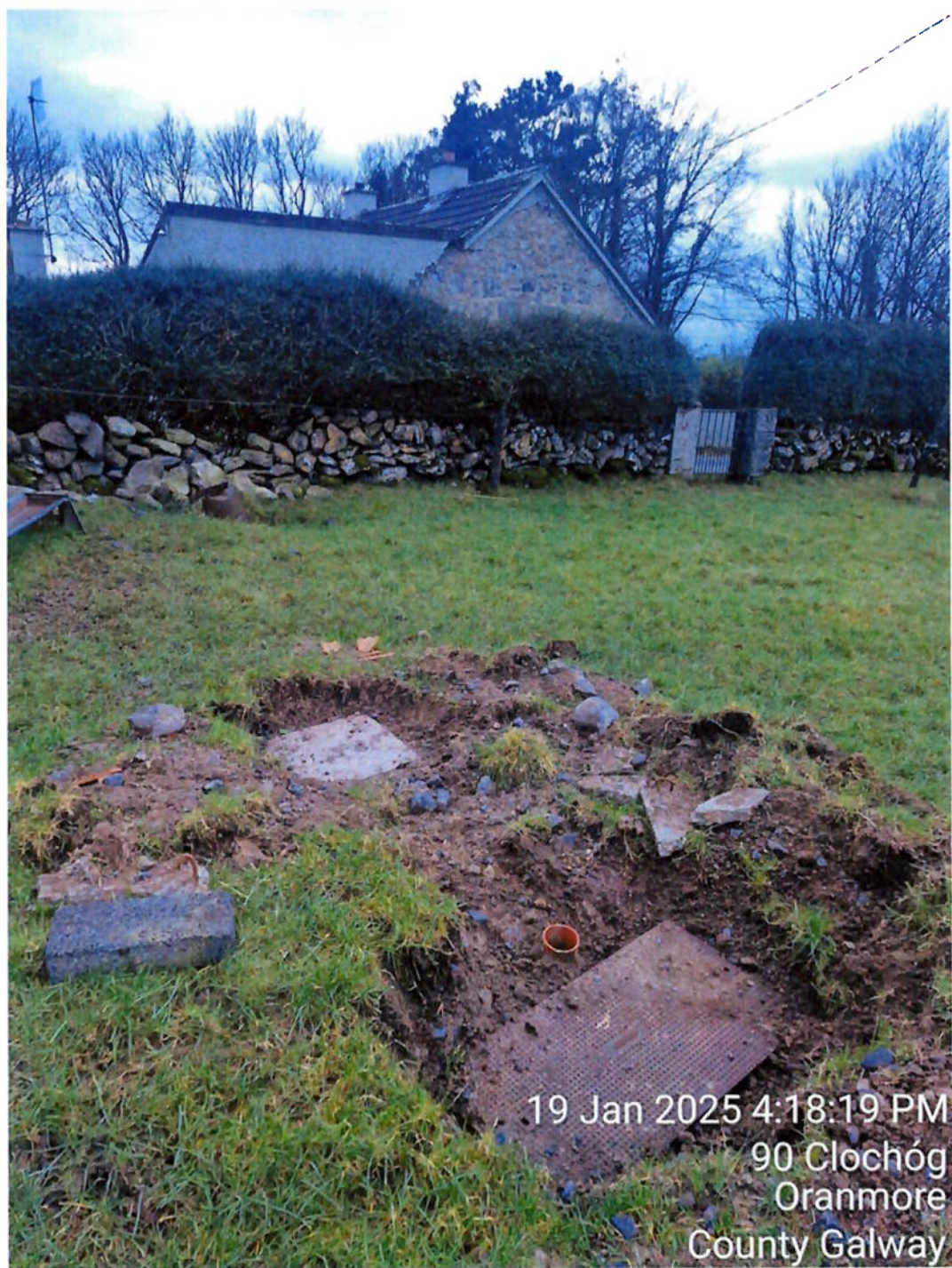
Fig 01. Photograph of exposed septic tank – location as per drawings
